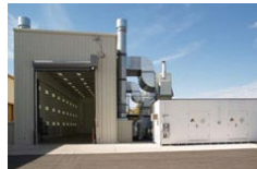
Outdoor Spray Booths
