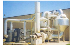
VOC Abatement Systems/Pollution Control
